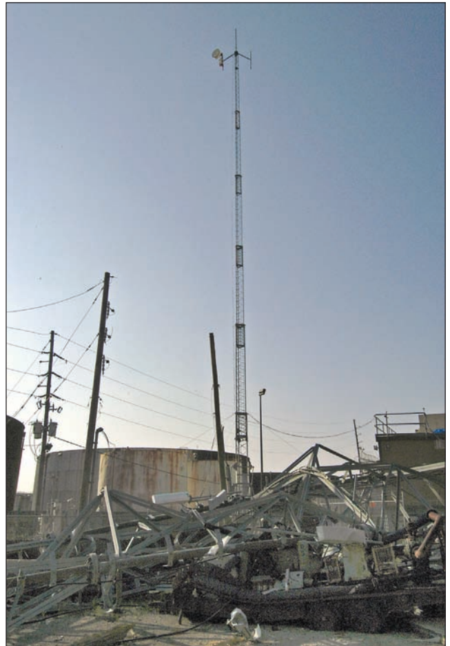
In the foreground lies the radio tower for the Jefferson Parish Sheriff's Office, destroyed by Hurricane Katrina. FEMA provided a National Communications System trailer-mounted portable communications tower 107 feet tall. Marvin Nauman/FEMA photo.
