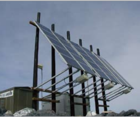
Control Point 2400 Watt Solar Array 15 Day Reserve Northern Utah
