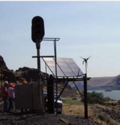
RR Intermediate Signal Installation 720 Watt Solar Array / Wind Hybrid Generator Back-up Southern Washington State
