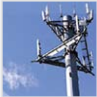
Base Station Infrastructure
