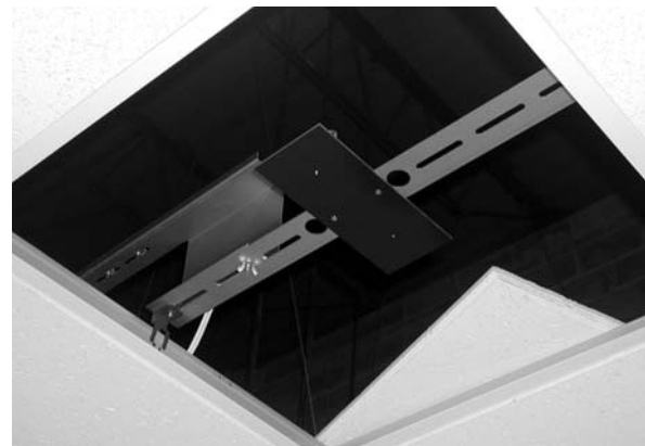
UFODAP1200 installed above ceiling (AP not shown)
